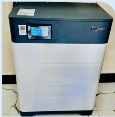
Figure 12: Solar power system
