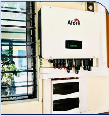
Figure 11: Solar power system
